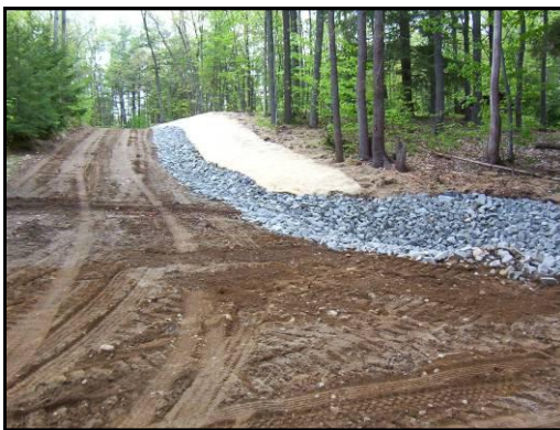
Camp road undergoing reconstruction. Road has been regraded to direct runoff to rip rap drainage ditch / detention structure along road side and new grass strip has been installed for soil stabilization.
